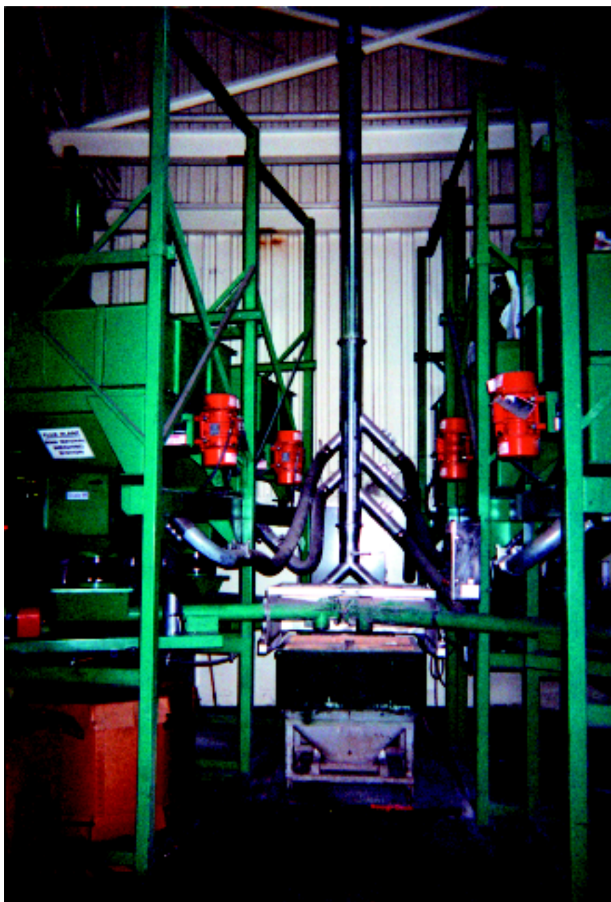
The five bulk bag unloaders and five volumetric screw feeders accurately feed material to a centrally located portable hopper.
